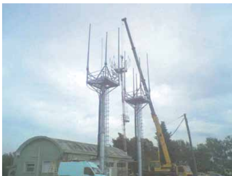
Pisa Airport Installation
